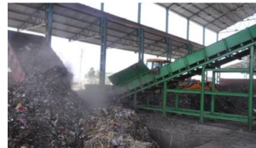
Kanpur Integrated Waste Management Facility
